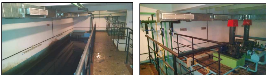
On-Site STP for treating waste water
