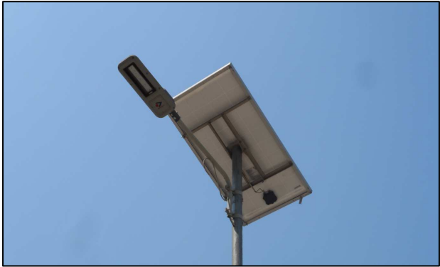
Stand Alone Solar-PV Street Lights
