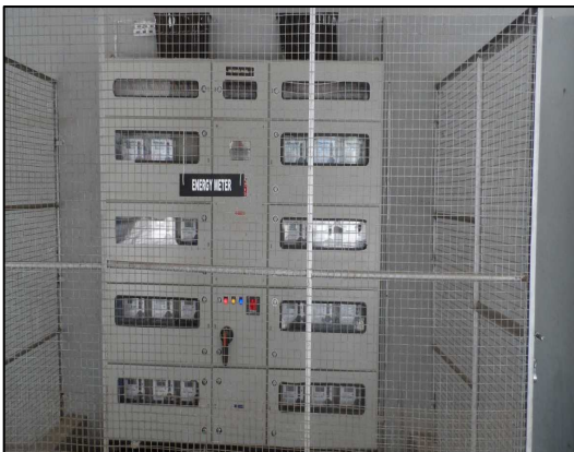
Energy Meters measuring Common Area Loads
