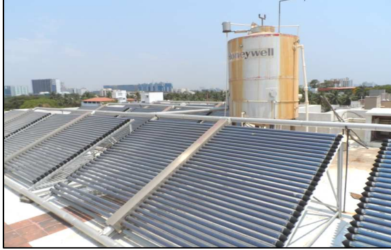
Centralized Solar Hot Water System
