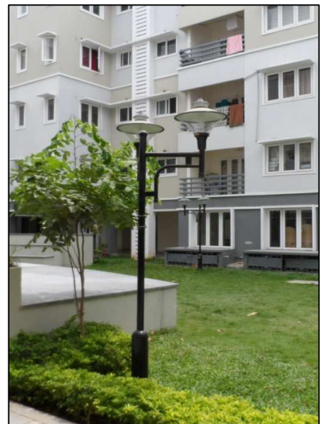
Covered Dome Light Fixture
