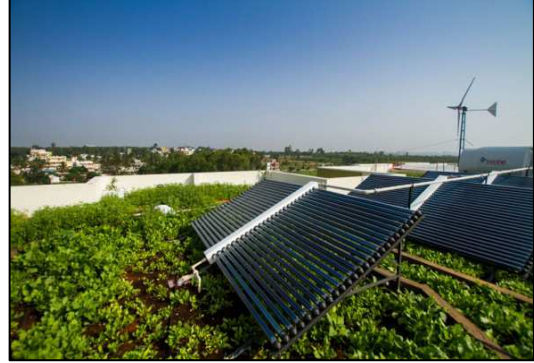
Individual Solar Hot Water System
