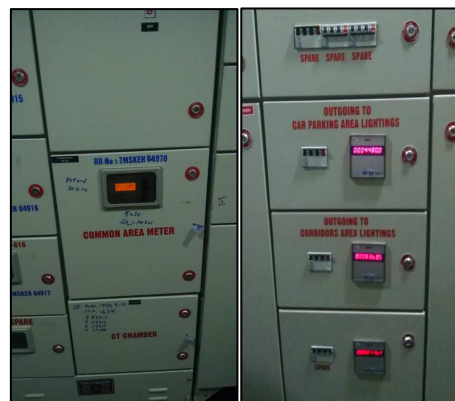
Energy Meters measuring Lighting and Equipment Loads
